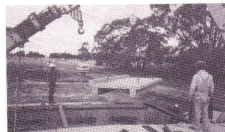
A Bridgette Plank is about to be placed on its rubber pads. Piers are held precisely in position by temporary struts, and small steel protection angles guide the slab gently into place.
