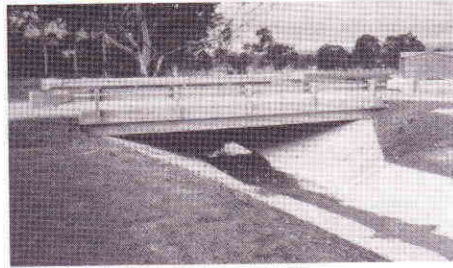
Access to a recreation reserve near Traralgon was constructed quickly and cheaply with 3 Bridgette planks 8.8m long, resting on simple footings.
