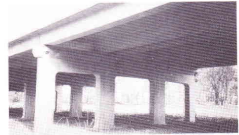
Underneath view showing the neat uncluttered appearance of the double-Tee section Bridgette planks.
