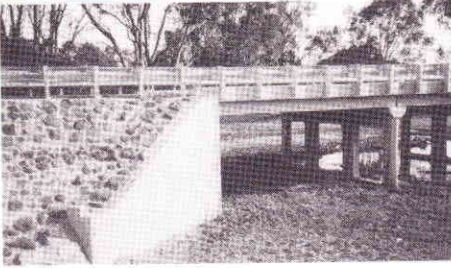
Stone beaching neatly laid by Lockhart Shire Council provided a functional and attractive finish on this Bridgette abutment.
