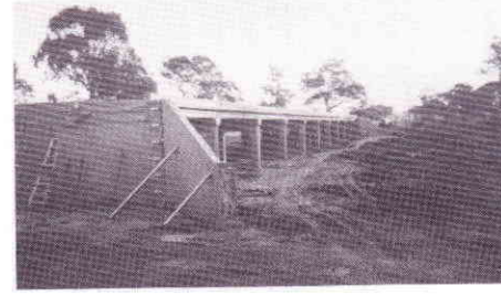
A double-lane Bridgette near Lockhart comprising 10 spans x 6m with abutment walls 3.3m high. Simple spread footings were constructed in less than two weeks, followed by erection of the superstructure which took about the same time.
